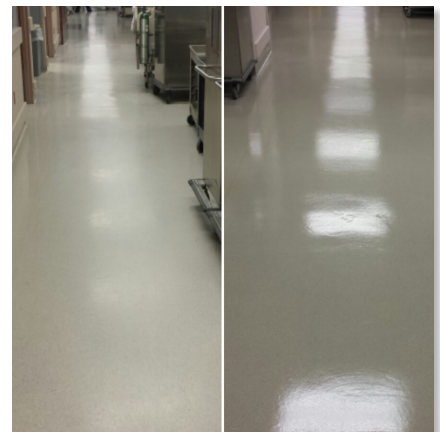
Linoleum Flooring Coated With X-PROTECT Vinyl & Linoleum (Jewish Hospital O.R., Before & After Comparison)
