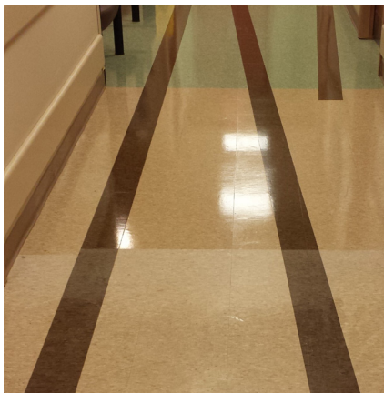
Linoleum Flooring Coated With X-PROTECT Vinyl & Linoleum (James A. Rhodes Hospital, Before & After Comparison)
